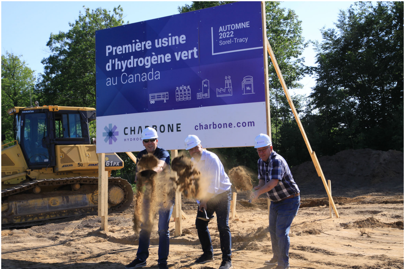
Left to right: S. Dallaire, CFO/ D. Gagnon CEO and Chairman of the board/ D. Charette COO First shovel – Courtesy of CHARBONE Hydrogen Corporation
